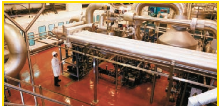
Investment in new pumps at a yeast production facility has increased efficiency
