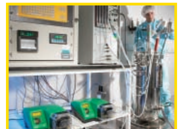
Two of the fifty pumps employed in fermentor feed for test kit production
